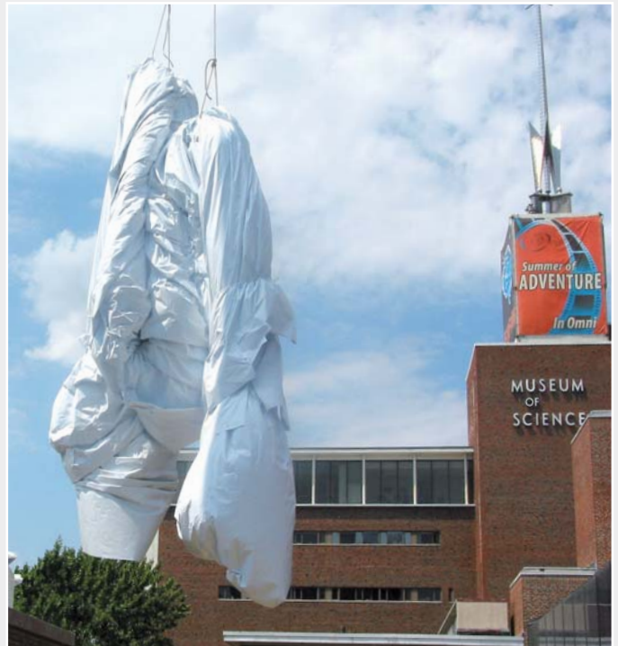
Hauling up the entire wrap from the flat roof top onto the dome.
