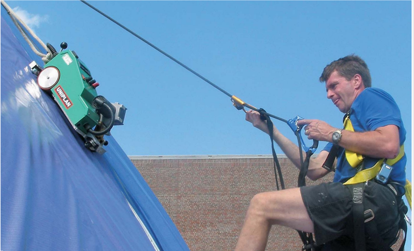
David King controlling the roll down of the UNIPLAN E for the final welding.
