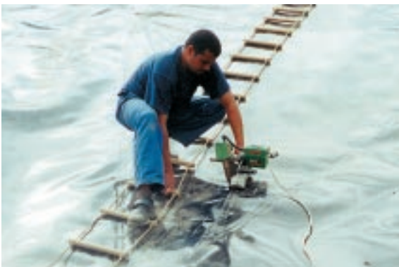
TWINNY T with test channel welding 1.5 mm PE-HD liners in a landfill.
