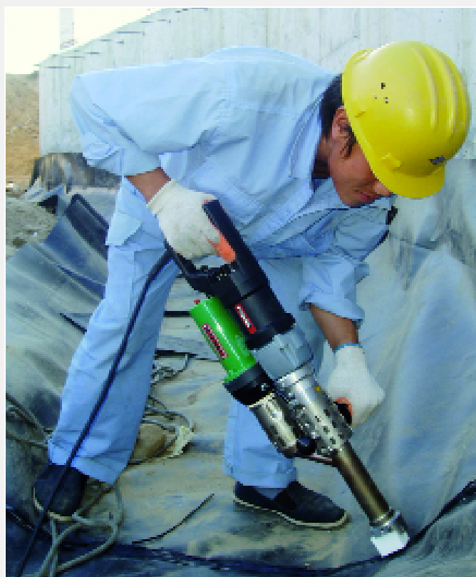
Extruding the sealing sheets on uneven subsurface with the FUSION 3 hand extruder.
